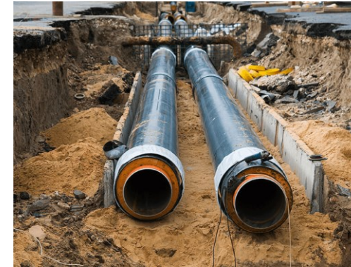
Supply and return pipe of a district heating network. These are pre-insulated pipes installed approximately 1-1.5 metres deep.
