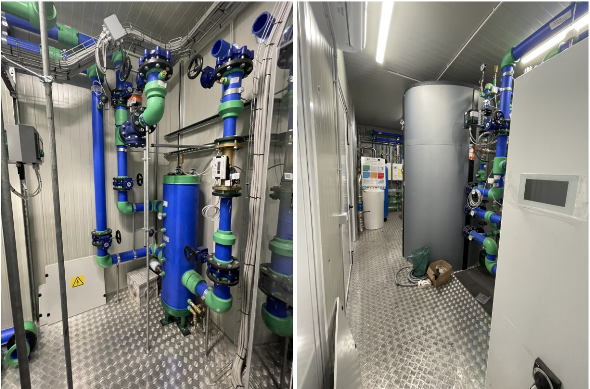
Figure 25: containerized geothermal plant after positioning (roof mounting).
