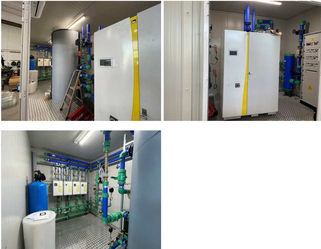
Figure 23: construction works at the containerized geothermal plant (tank, heat pump, sanitary hot water fast heat exchangers). Pictures taken during container prefabrication at Termotecnica Sebina.
